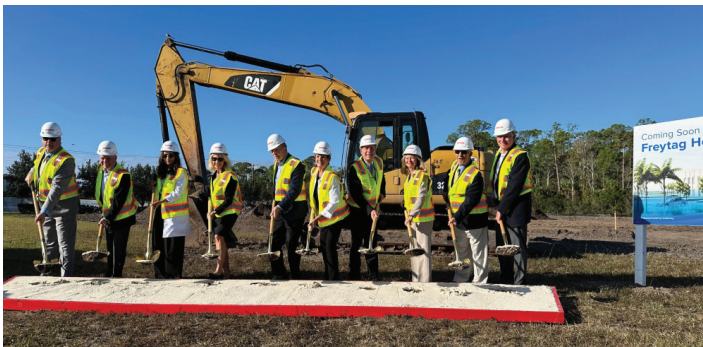
AdventHealth Palm Coast broke ground on construction of the Freytag Health Plaza recently. Named in honor of Palm Coast residents Peter and Sue Freytag, the Health Plaza will become a vital hub for cancer treatment, primary care and rehabilitation services.
